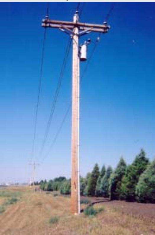
Providing power to new housing developments north of Bismarck, Capital Electric has installed numerous 35 ft. cedar distribution poles to keep up with new construction.
