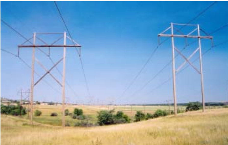
New 115kV transmission lines with 85 ft. cedar poles were built last year to increase capacity. These lines extend north from a generating station north of Bismarck.
