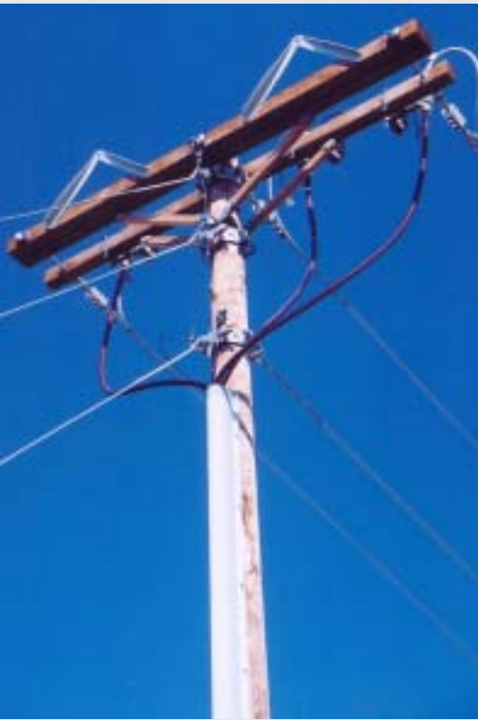
To provide raptor protection, Mountrail Williams has retrofit their system by adding triangular shaped devices on poles where connections occur, and by increasing crossarm length to 10 ft.
