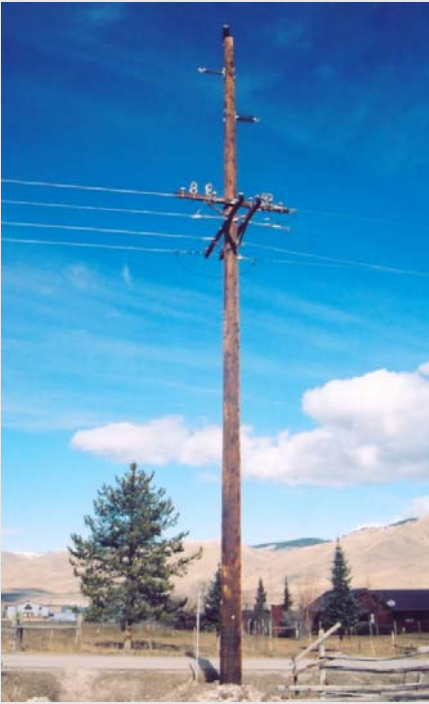
The Jocko Line north of Arlee, MT uses 65 ft. and 70 ft. Class 1 cedar poles on a 69kV line that began installation in February for that portion of the U.S. Highway 93 widening project .
