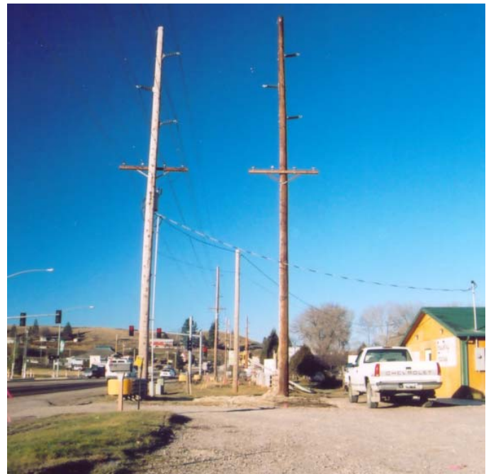
Here, new 70 ft. Class 1 cedar poles were installed along side the older lines on State Highway 35. This line stretches from a substation at Polson, MT to U.S. Highway 93, allowing for future widening of that roadway.
