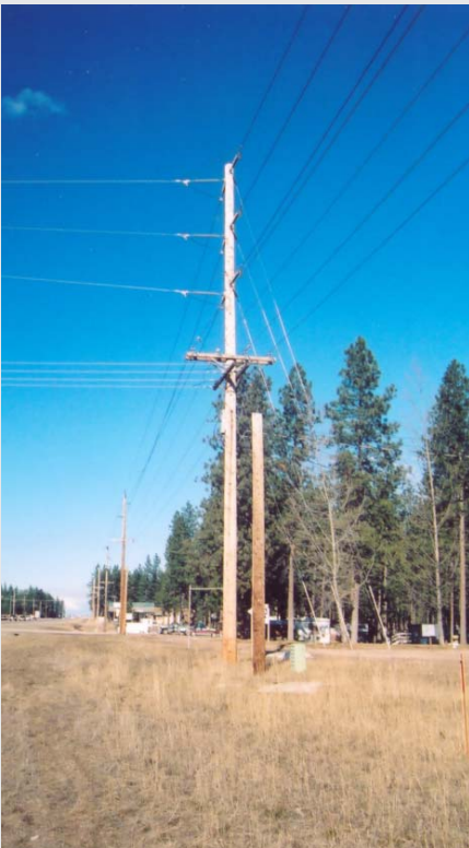
Near the Mission Valley Power office at Pablo, MT, 60 ft. Class 1 cedar poles carrying 69kV are being used for the U.S. Highway 93 widening.
