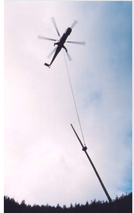
Above, this "Sky Crane" helicopter lifts a Western Red Cedar log from the forest and transports it to a nearby logging road. Light weight cedar poles are an ideal species for helicopter logging.
