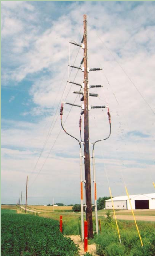
This newly constructed six-mile line using 70 ft. cedar poles serves a new ethanol plant in Granite Falls, MN. To pass under a transmission line in the area, the new line was put underground for 80 ft.
