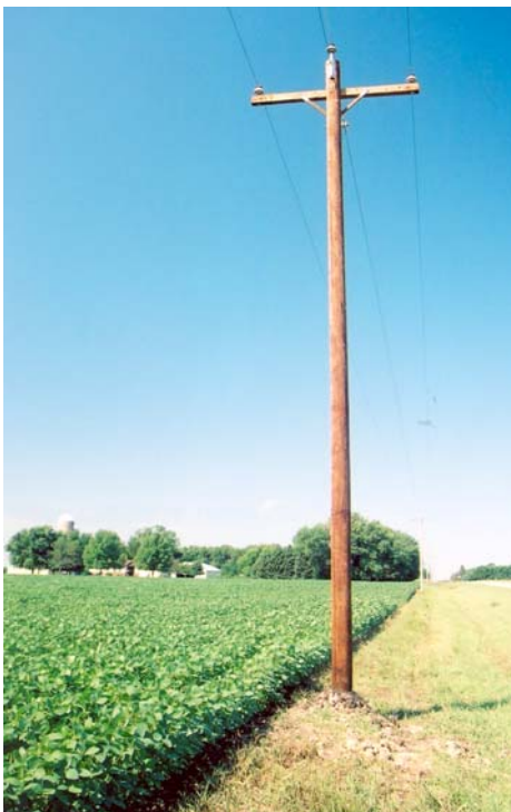
Kandiyohi Power upgraded and replaced cedar poles to a three-phase line with new Class 5, 35 ft. cedar poles on this line near Prinsburg, MN.
