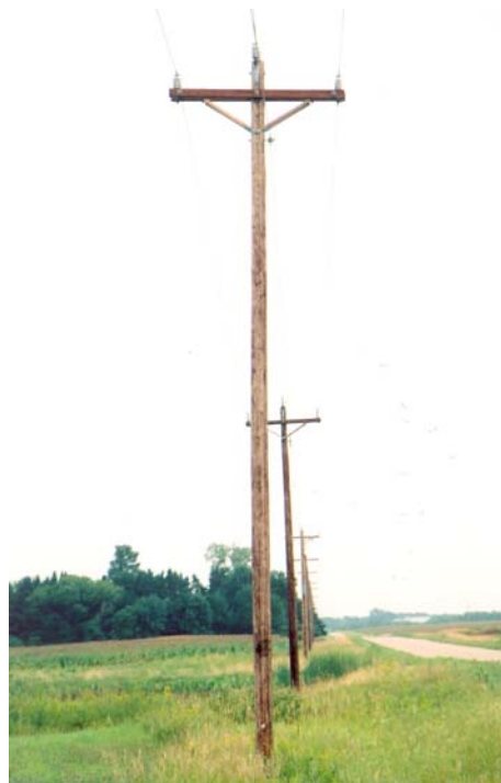
A recent project, this new 1.25 mile cedar Atwater line was constructed by Kandiyohi Power to replace a line on private property. These Western Red Cedar poles are Class 6, 35 ft.
