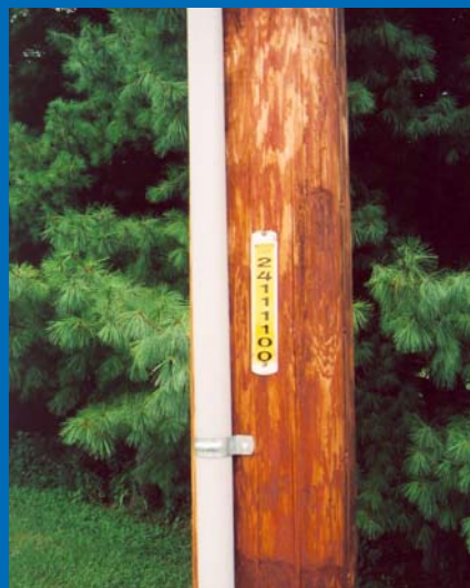
All poles in the Meeker Coop system are tagged like this pole for easy identification in their GPS system.
