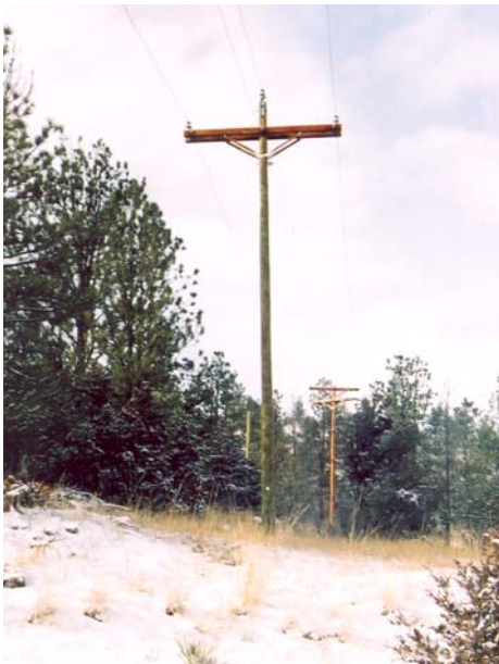
Due to a recent road widening and new bridge installation, this line at Reedspoint, MT, was installed using three-phase, 40 ft., Class 6 cedar poles for distribution.
