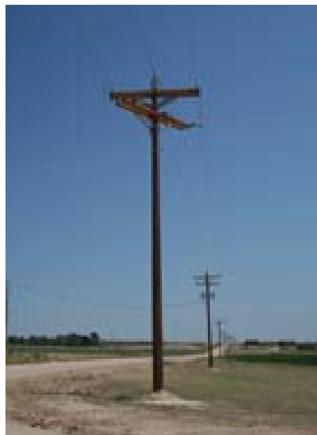
A new 40 ft. Class 6 cedar pole line was recently installed to provide power for irrigation of sugar beet, corn, alfalfa, and pinto bean crops.
