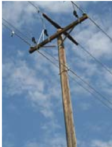
When new cedar poles are placed in service they are equipped with raptor protection, including the device shown here, as well as a ten ft. crossarm.
