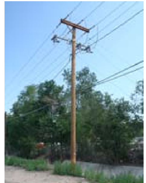
This 50 ft. Class 4 cedar poles carries double circuit 12.5kV and 7.2kV lines.
