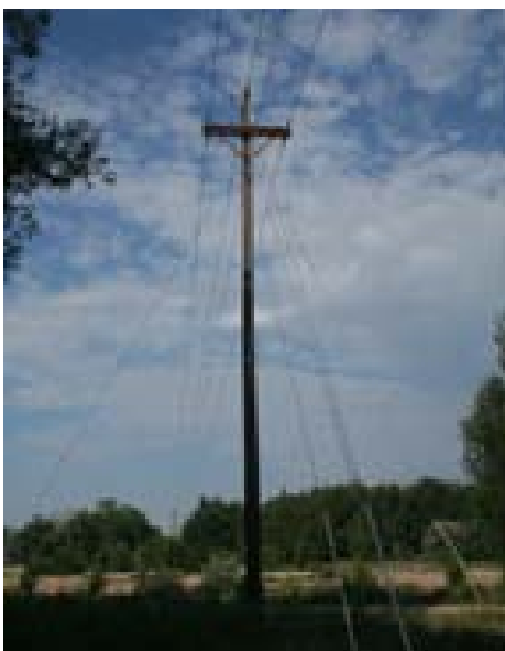
This line of 60 ft. Class 5 cedar poles carries a 12.5kV line across Monument Creek.
