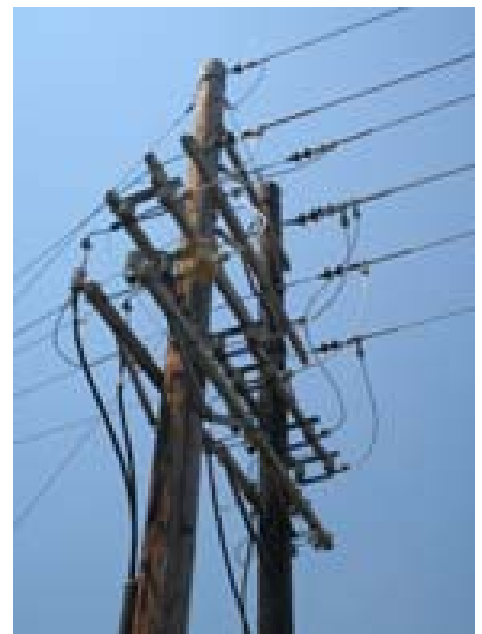
Many of the Morgan County REA lines have been re-cabled to increase capacity. On this line, east of Brush, six heavy cables of 477 circular mills each are supported on Western Red Cedar poles.
