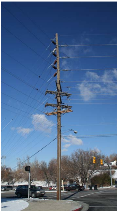
This three-line junction on a 75 ft. Class 1 cedar pole is near Brigham Young Univ., the largest electrical user in the Provo City Power system.
