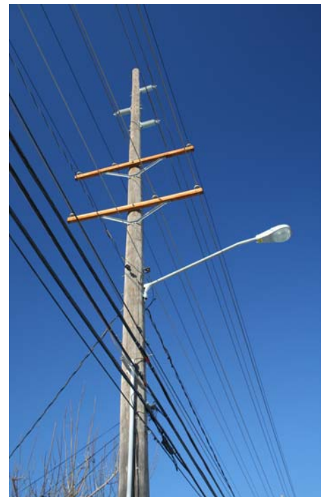
Forty-two miles of transmission line surround Provo, and is built with 70 ft. Class 1 cedar poles. Distribution lines are also carried on these poles along with considerable cable underbuild.
