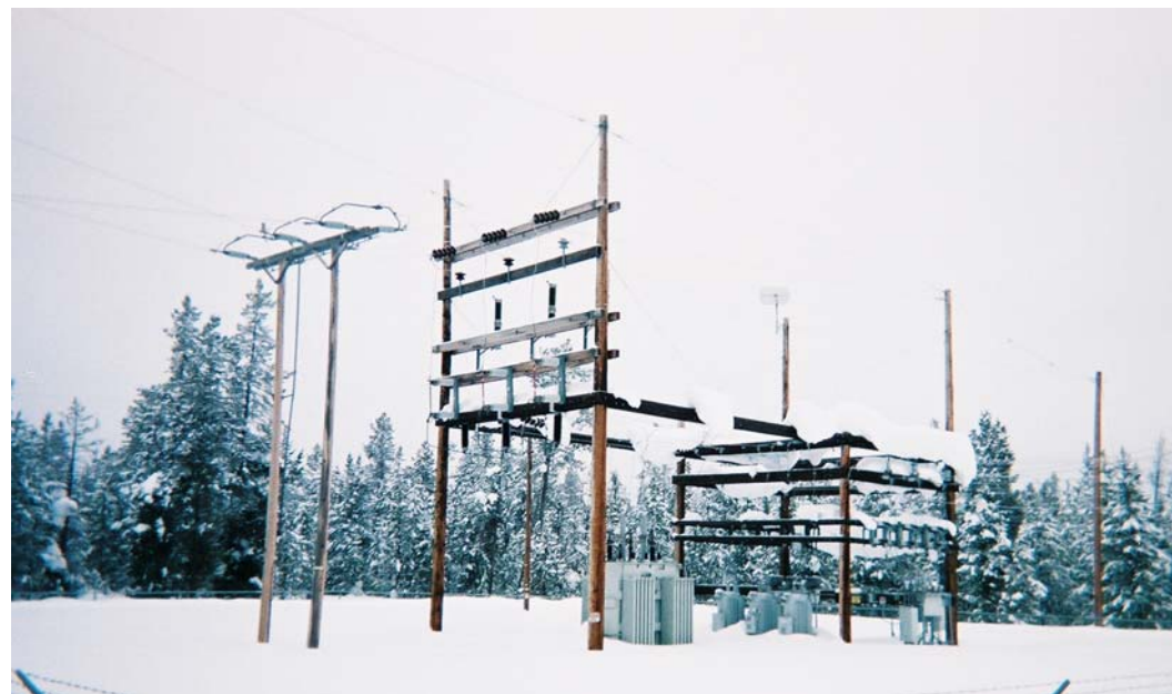
Using 50 ft. full-length penta treated cedar poles, this Fall River Electric substation between Ashton and Yellowstone Park was built in 1966.
