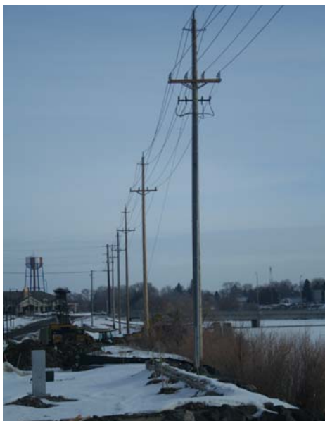
This line was built along the Snake River uses 85-ft. H-1 cedar poles to raise the height of the wires so the office building to the west would have an unobstructed view.
