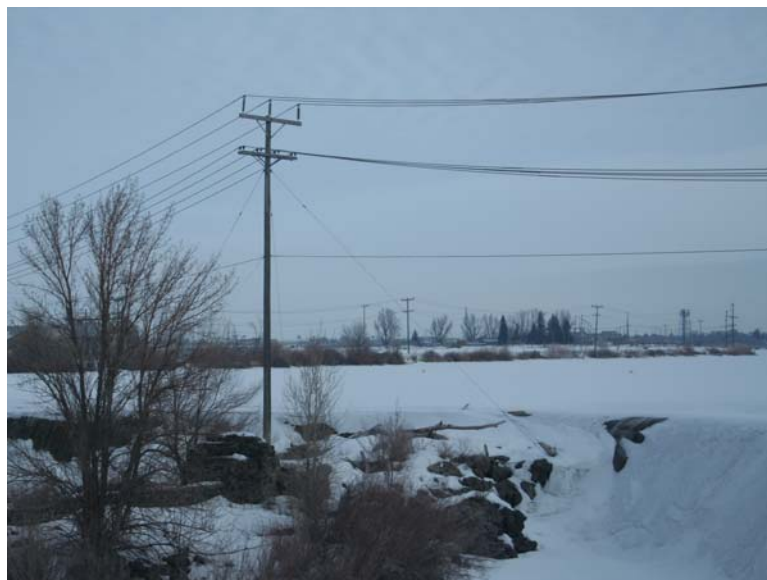
A 600 foot crossing of the Snake River, this line is scheduled to be rebuilt this year with cedar poles.
