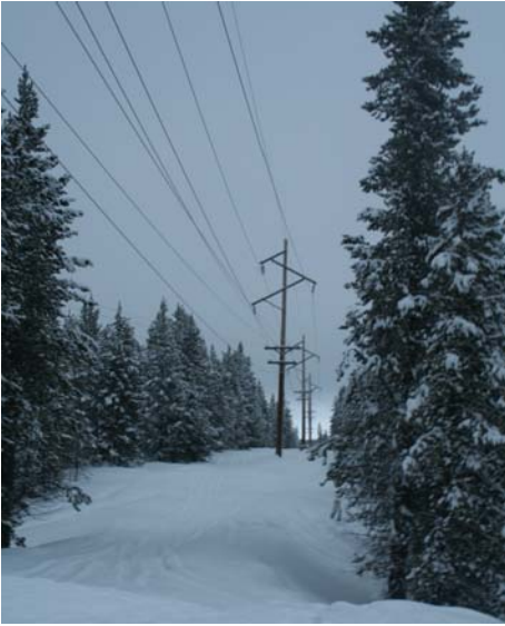
This line, built in 1999 with 75 ft. cedar poles, delivers power to customers near Yellowstone National Park.
