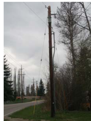
This a typical 35 ft. Class 5 cedar distribution pole used in the Flathead Electric system.
