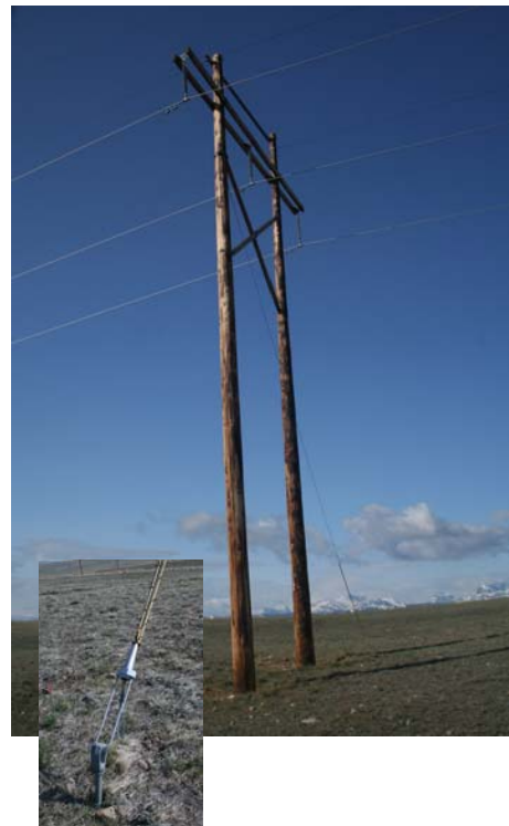
Sustained high winds in the Glacier Electric system can cause vibration that “walks” a pole structure out of the ground. The utility solved this potential problem by guying H-frame structures at right angles to the line direction. The cedar poles in this line are 70 ft. Class 2.
