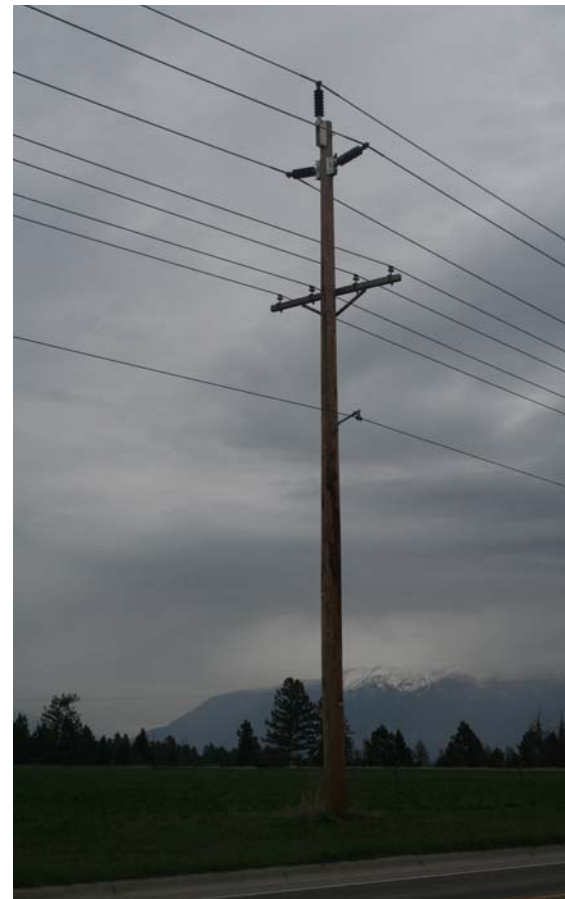
A typical Flathead Electric line, this line carries 34.5kV transmission at the top, 17.2kV distribution in the middle and cable below. A recently rebuilt line, these cedar poles are 55 ft. Class 1, full-length, penta treated.
