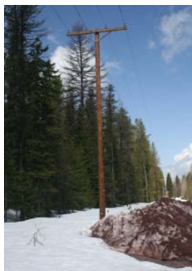
This 45 ft. cedar distribution pole carries 14.4kV power into the Rocky Mountains along Hwy 2.
