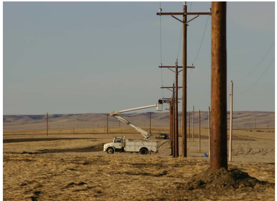
Twelve miles of new 70 ft, Class 1 cedar transmission line was constructed in 2007 by Moreau-Grand Electric. This along with a new substation and 15.2 miles of new cedar three-phase, supply power to a new water intake for the Mni Waste water project that brings safe drinking water to Dewey and Ziebach Counties.
