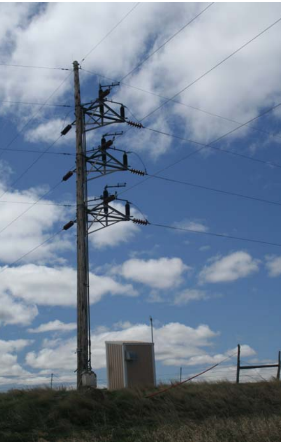
This 45 ft. pole is typical of West Central Electric Coop's service to rural users in the Murdo, SD, area.
