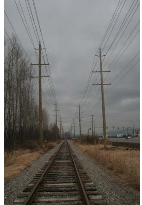
These recently constructed 138kV double transmission lines use 65 ft. cedar poles and transmit power from Abbotsford to Mission, BC.
