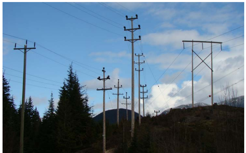
Below, several Western Red Cedar lines leave the Burrard Station. The H-frames use 75 ft. poles, and the other poles are 50 ft. to 65 ft.
